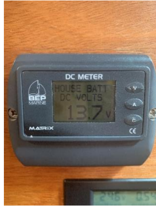
AC Volts and Current Meter
